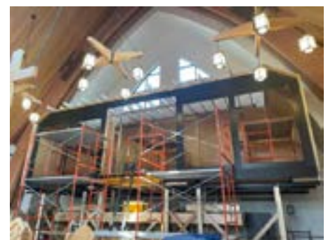
The pipe organ project is both massive and intricate, interesting to watch, and nearly complete!
